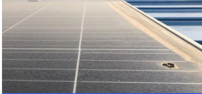
Pollutants such as mud and bird droppings seriously affect system efficiency
